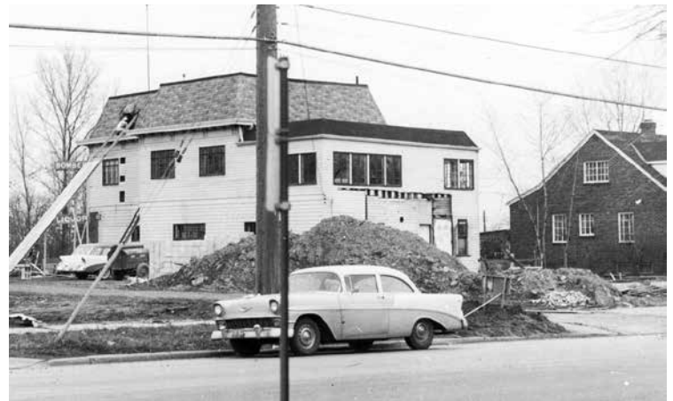
In this 1957 photo, workmen are remodeling the old Rockport House/Bomber Tavern which has been moved from its original location and is now one lot to the east on Puritas Avenue. Cleveland Public Library Collection.
